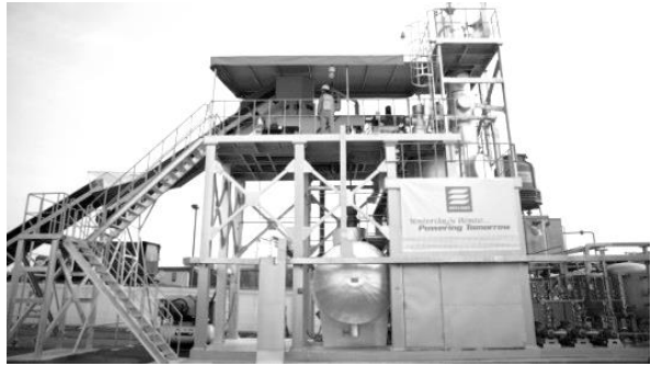
A plastic-to-oil processing plant. It is not only a simple process but a viable supplement for gasoline and diesel.
